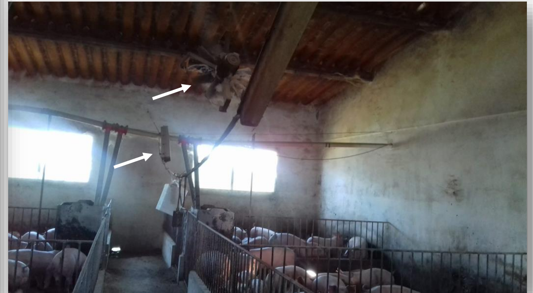
A bad maintenance of the electrical system may lead to accidents
